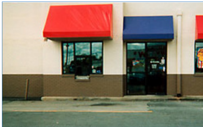
Scott fell on the sidewalk near the down spout.
